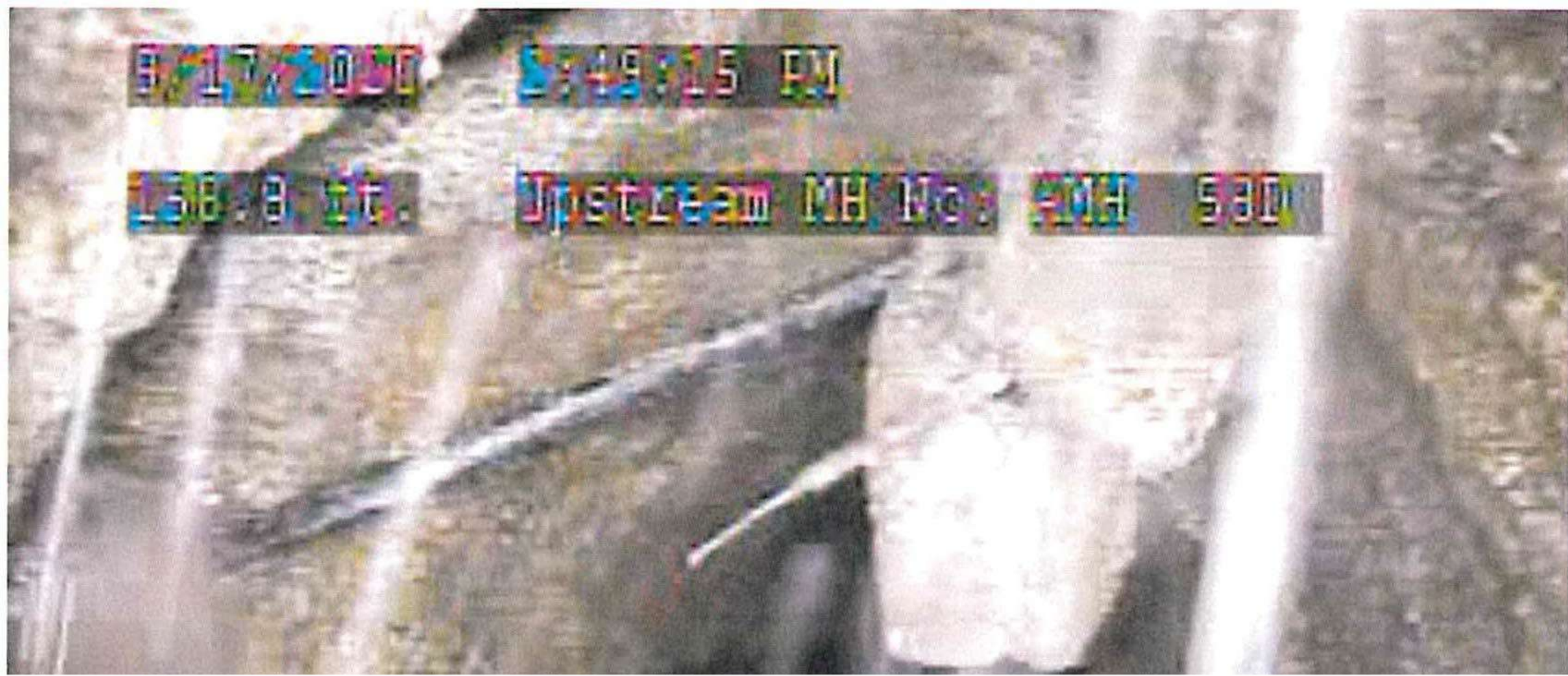
Current Condition of Collection System Hole and Re-Bar Visible Behind Pipe
